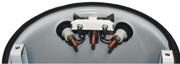
The spark gap mounted internally on the LV neutral bushing with the electrodes connected to the X1 and X3 bushings.
